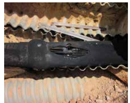
➤ Cable fault, 1-core 11 kV joint failure
