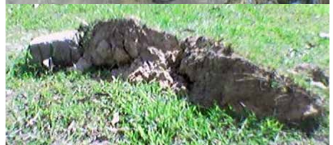
➤ exploded 132 kV joint after cable fault, 132 kV XLPE, explosion lifted soil above the faulty spot.
