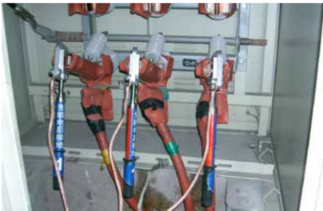
➤ Grounding of all phases
