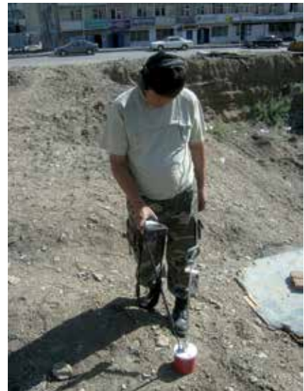
➤ field application acoustic fault location
